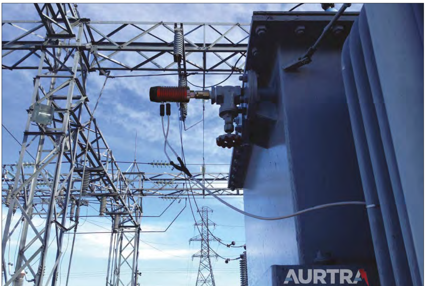
Figure 3. Aurtra HealthSense Sensor installed in top fill valve
