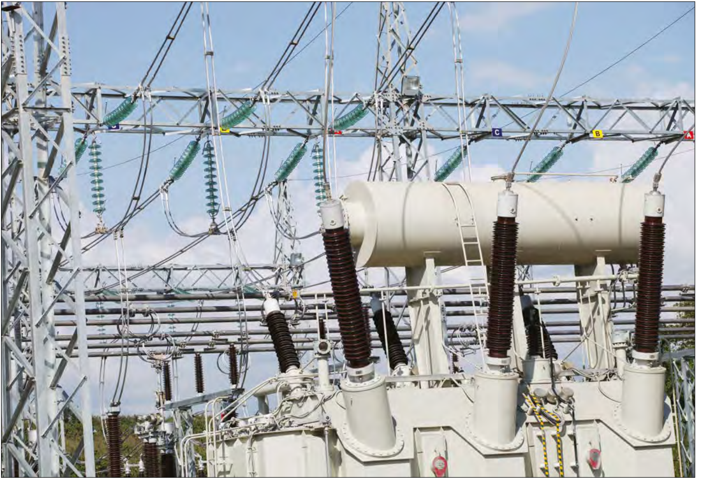
Figure 4. Power transformer bushing
