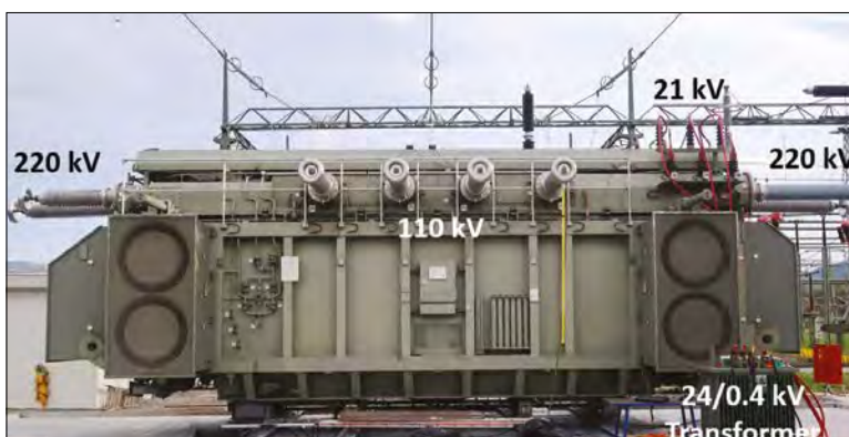
Figure 1. View of the 300 MVA transformer
